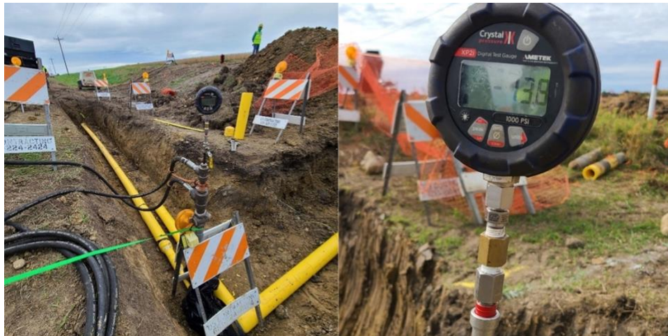
Figure 19: Pressure monitoring tree installed on pipeline
