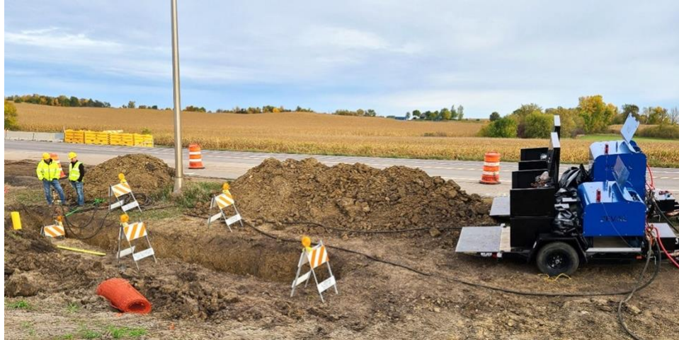
Figure 18: Equipment setup at site
